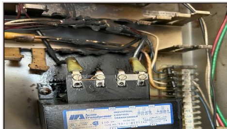
Burnt Transformer — Controller
